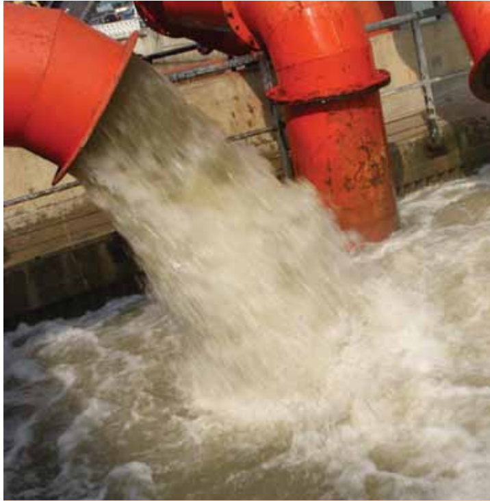
This summer the Oldham County Sewer District repaired and upgraded the sewer system and made improvements to wastewater plants.
