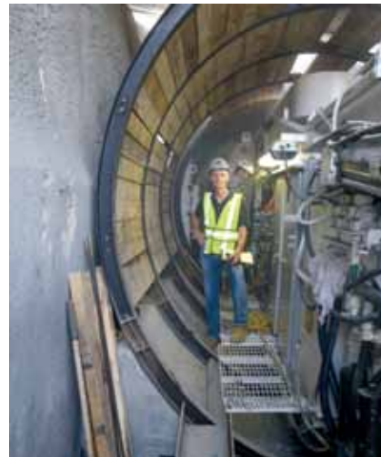
Crews work around the clock on the 12-foot wide, 6-mile long wastewater conveyance tunnel.
